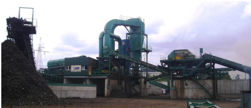
Fig. 57. Shredding installation of Centrozlom S.A.
