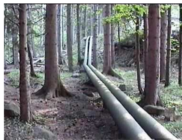
Fig. 3.4. Feeding pipes of SHP.
