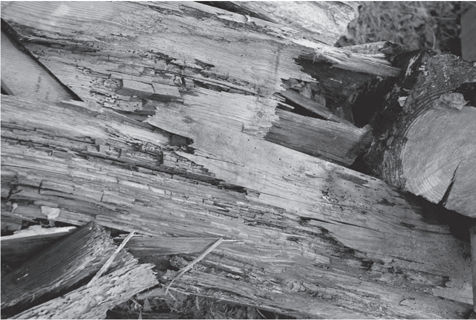
Fig. 1. Fragment of the destroyed roof framing construction
