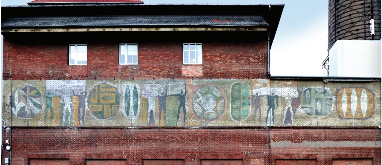
Fig. 12. Building of the switching station of sections P1-4 and P-7 (new electrical switching station from 1917–1923) on the south side, the wall with a mural by T. Ciałowicz from the late 1960s (photo by A. Gryglewska, 2019)
