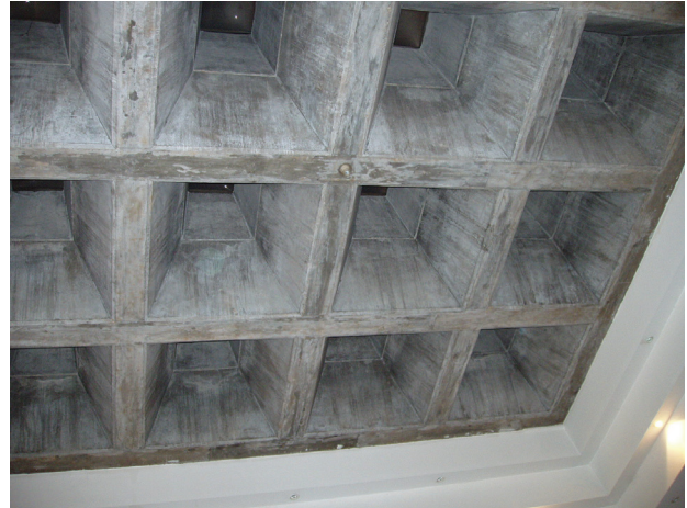
Fig. 10. Altuğ and Behruz Çinici, METU Faculty of Architecture Building in Ankara – the concrete ceiling (photo by W. Niebrzydowski)
