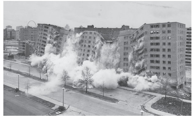
Fig. 3. Demolition of Pruitt-Igoe housing complex on March 16, 1972. Simone Brott notices the similarity in the form of the Dr Chau Chak Wing building to the moment captured in this photo (photo by U.S. Department of Housing and Urban Development, public domain, via Wikimedia Commons, source: commons.wikimedia.org/wiki/File:Pruitt-igoe_collapse-series.jpg , accessed November 24, 2025, cropped by T. Omieciński)
