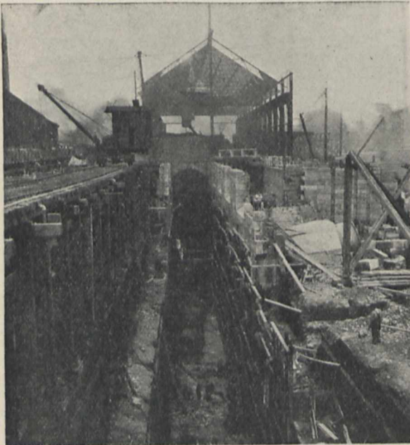
FIG. 2.—Power House of Canadian Niagara Power Co., being erected over the wheel-pit.
