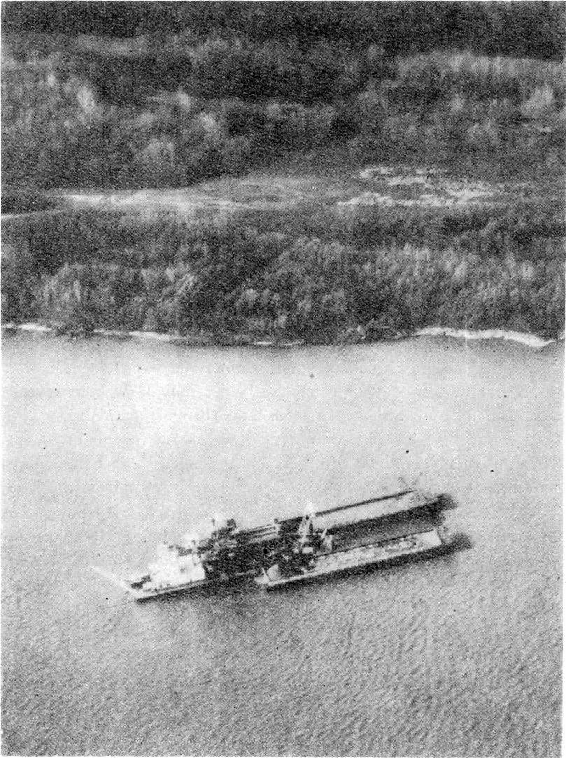
Fig. 3. Dredging and processing plant with two cargo barges located in the Ohio river. (No visible plume was detected beyond 30 m downstream from the discharge)
