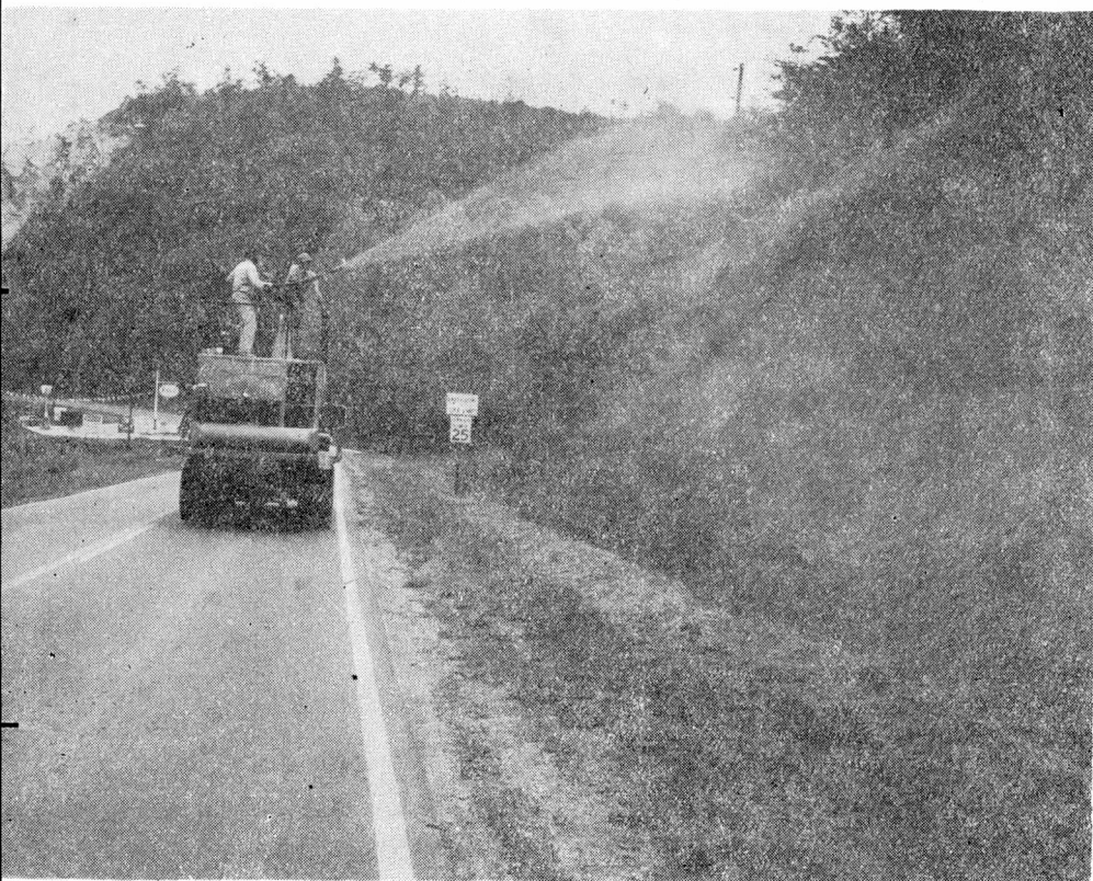
Fig. 5. Hydroseeding is one of the most effective methods of restoring protective vegetative cover on highly erosive areas
