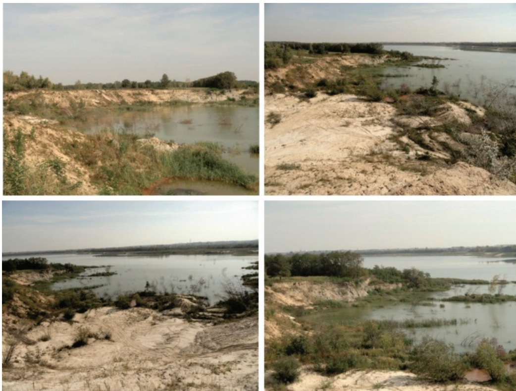
Fig. 1. State of the slope after the formation of the landslide (Source: photo by J. Jakóbczyk)
